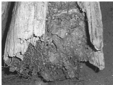
Fig. 4. Decayed, hollowed-out lower portion of a nineteenth-century, eastern-red-cedar post from the galerie of the Green Tree Tavern, Ste. Genevieve, Missouri.
