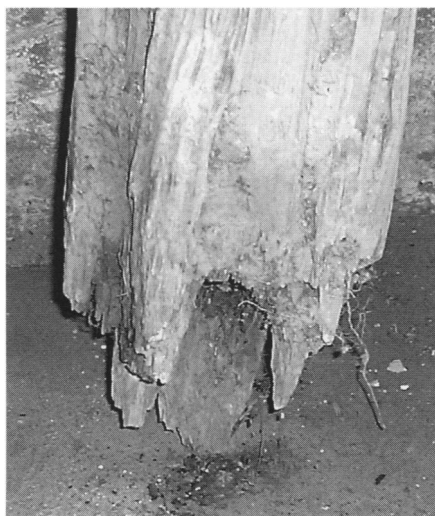
Fig. 5. Profile of a decayed eastern-red-cedar post.
