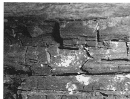
Fig. 3. Detail of fungal decay in an eastern-red-cedar post more than two hundred years old that has been removed from the ground.
